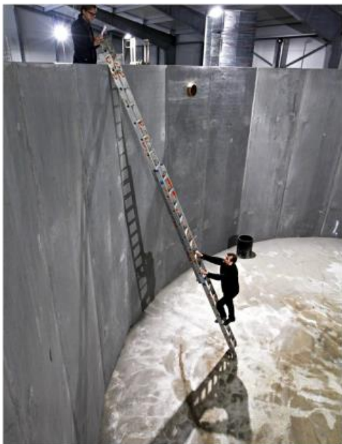
Figure 13: Large tanks at Langsand Laks RAS salmon farm in Denmark (Source Atlantic Sapphire)
